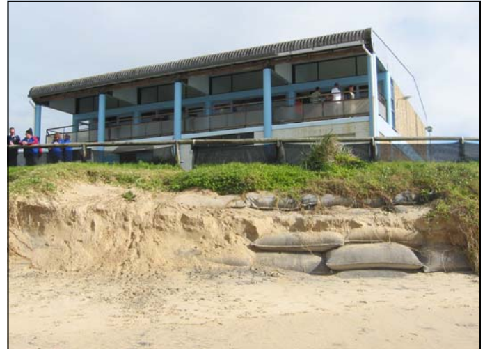
ELCOROCK® exposed after severe sea swells
