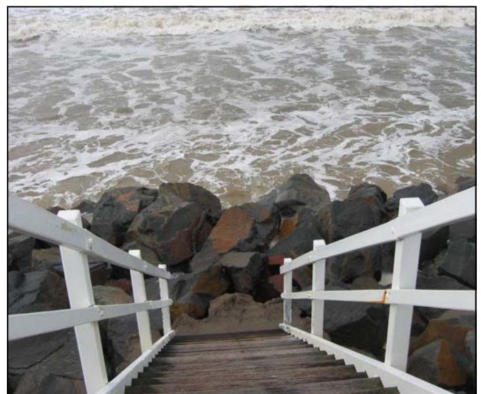
Displaced rock armour protection
